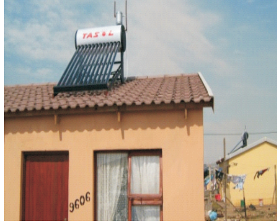
Figure 7: SWH installed at one of the houses participating in the Standard Bank Low Pressure Solar Water Heater Programme for South Africa
