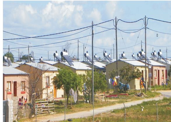
Figure 5 SASSA Low Pressure Solar Water Heating Programme
