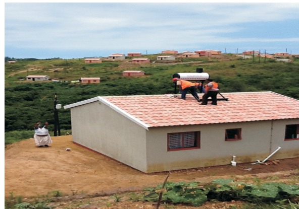
Figure 6: Installation of a SHW of the SASSA programme promoting access to services through free installations thereby improving livelihood.
